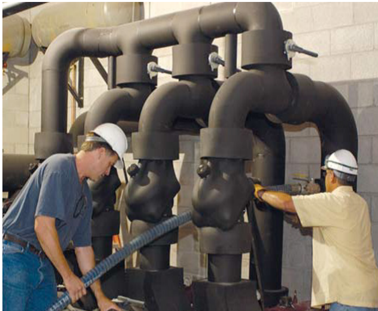
Daniel Laitila of Serve-Ice (left) and truck driver Bernie McClain (right) work together to fill high-performance DOWTHERM™ SR-1 Heat Transfer Fluid into the Midland Civic Arena ice refrigeration system.
