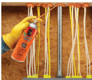
Electrical penetrations through floors
