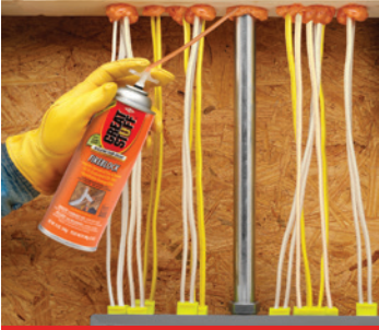
Electrical penetrations through floors
