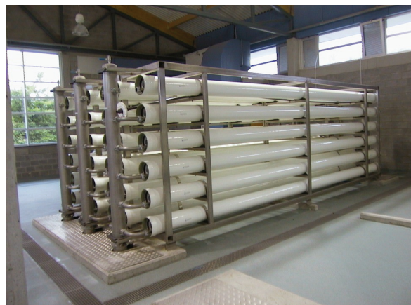
Pressure vessels housing reverse osmosis elements at the water treatment facility (Photo courtesy of Intermunicipal Water Company of the Veurne Region)
