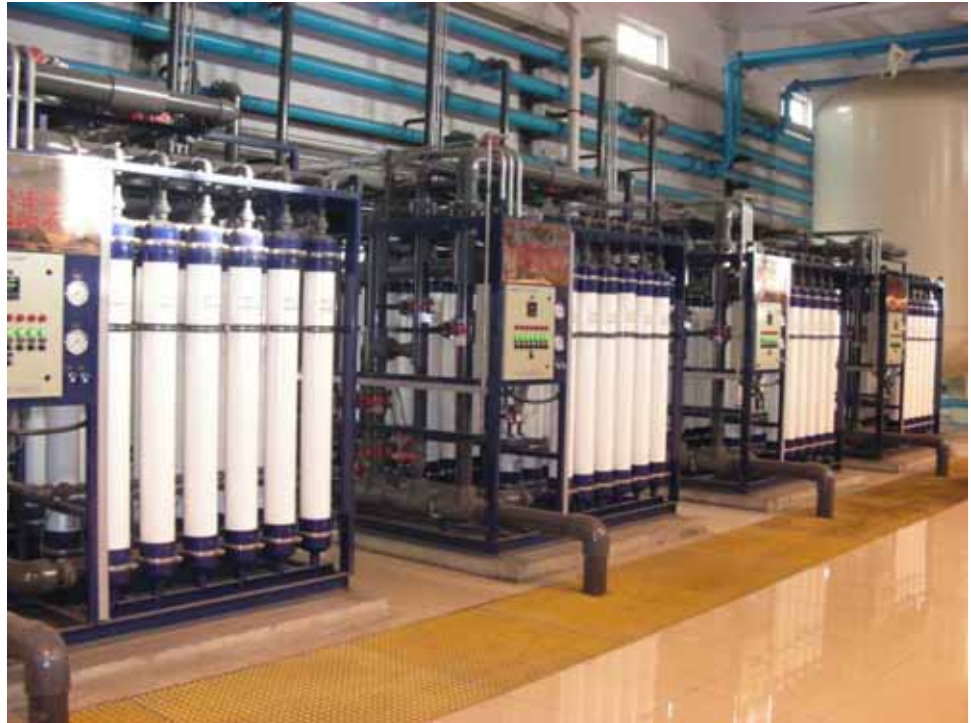
Ultrafiltration skids with DOW™ Ultrafiltration SFP-2660 modules in the ShanXi DaTong installation. (Photo courtesy of ShanXi DaTong Co-gen Ltd.)
