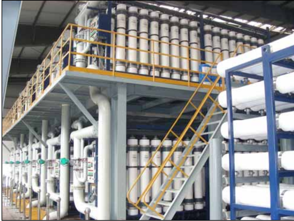
Two-floor arrangement of DOW™ Ultrafiltration SFP-2860 modules in the Taiyuan facility. (Photo courtesy of Taiyuan Steel Group Co. Ltd.)
