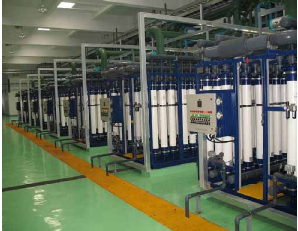
Skids of DOW™ Ultrafiltration modules in the HeBei facility. (Photo courtesy of HeBei DaTang WangTang International HuaTan Electricity Co. Ltd.)
