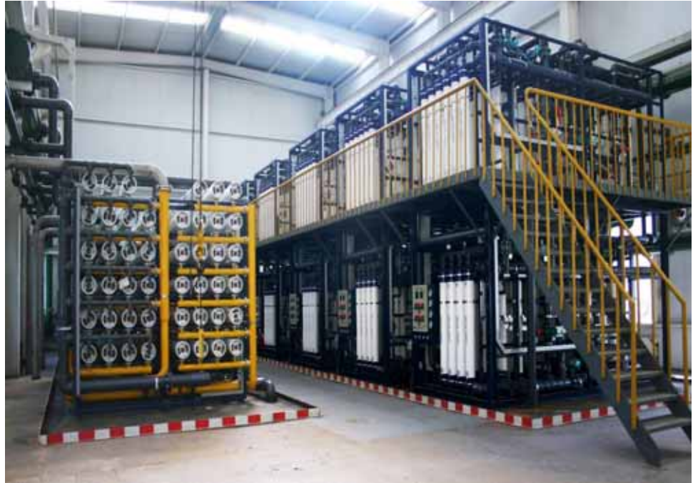
DOW™ Ultrafiltration modules in the YanShan facility are stacked via a mezzanine in an efficient, space-saving design. (Photo courtesy of Beijing YanShan Petrochemical Co. Ltd.)
