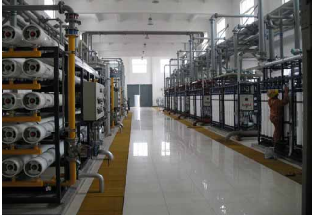
DOW™ Ultrafiltration and FILMTEC™ reverse osmosis installations at NingBo facility. (Photo courtesy of NingBo Jiufeng Co-gen Ltd.)
