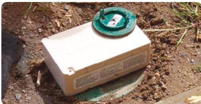
Picture 9: SMAG (Soil Mounted Above-Ground station)
